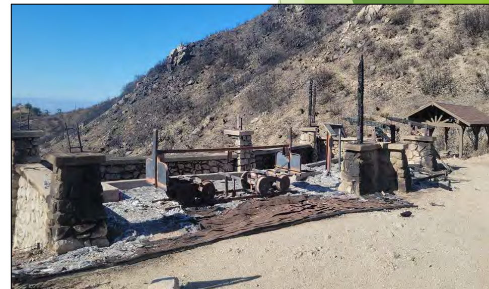
ation Point Pavilion Burned Structure
